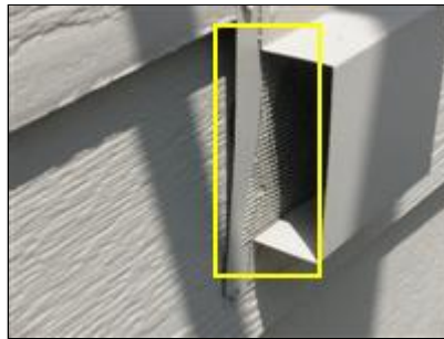
9.3 Picture 1 Vent for fireplace
