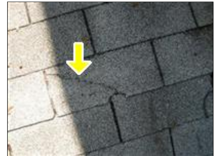
1.0 Picture 3 Cracked shingles
