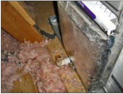
9.0 Picture 1 AC unit in the attic
