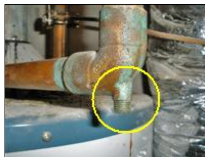
8.6 Picture 2 Discharge line of T &amp; P valve
