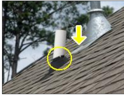
1.2 Picture 1 Waste vent boot and flue
