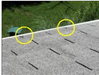
1.0 Picture 2 Exposed nails
