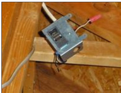
6.4 Picture 1 Loose wiring box in attic
