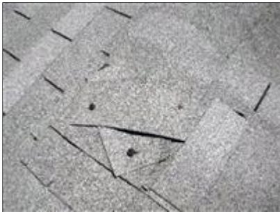
1.0 Picture 1 Exposed nail heads
