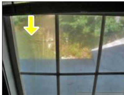
10.4 Picture 1 Crack in window
