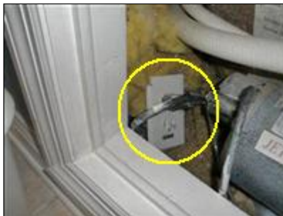
6.5 Picture 1 GFCI outlet
